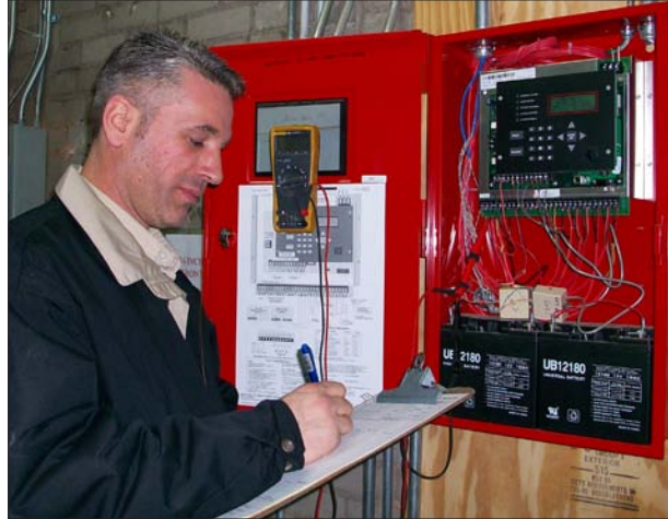
Technician, Mike Parenteau, inspects a fire alarm panel. Preventative maintenance can help reduce false alarms and emergency service costs.
